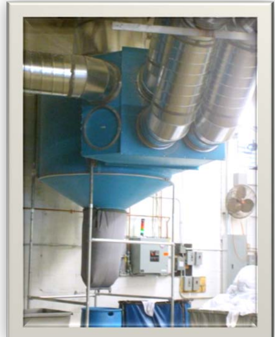
AFTER Inside view of Model DLF – 530 and mutiple dryer hook-ups NEW QEI Greenheck Fan on the roof
