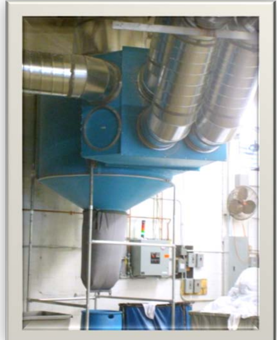
AFTER Inside view of Model DLF – 530 and mutiple dryer hook-ups NEW QEI Greenheck Fan on the roof
